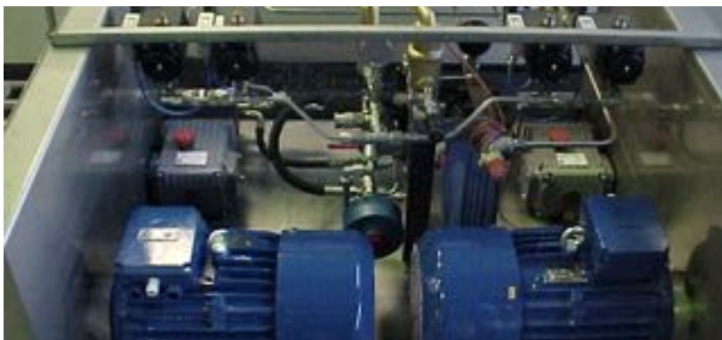
Redundant pump station
